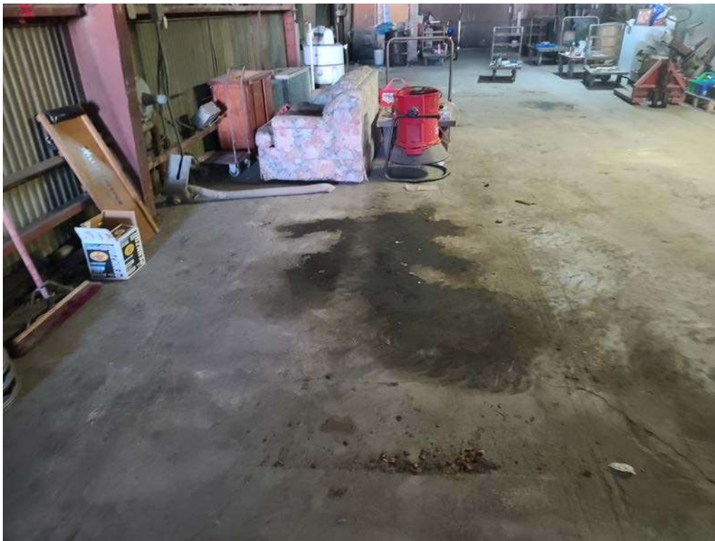
Photo 13: View of surficial staining in building.
