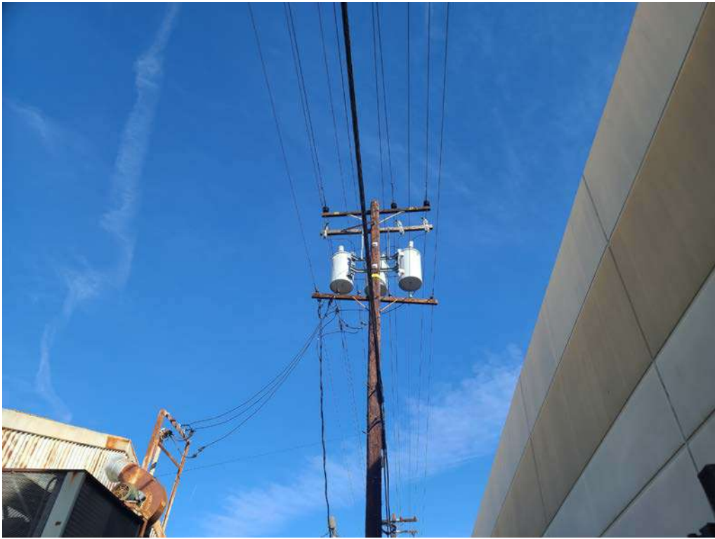
Photo 17: View of pole mounted transformers.
