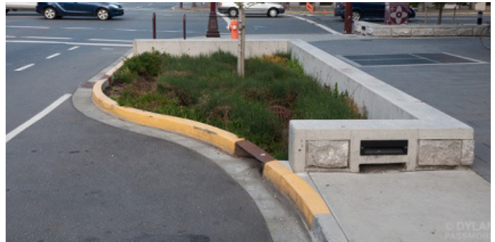
Bioswale within a curb extension also provides seating.
